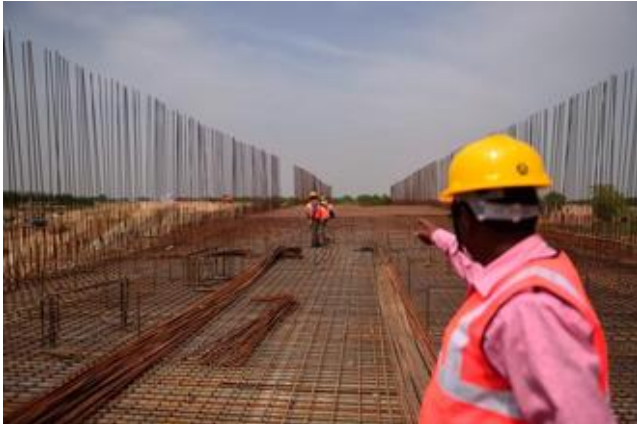
Eastern Peripheral Expressway under construction in Mohana village of Faridabad, Haryana. Photo: Pradeep Gaur/ Mint
